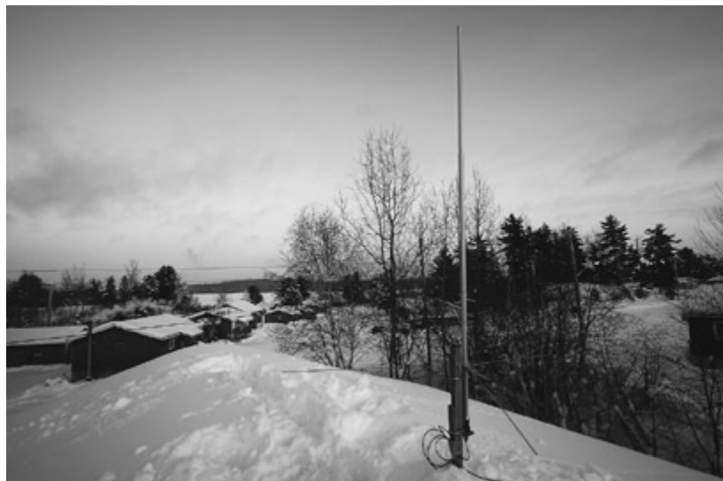
Antenna at Radio Barriere Lake
